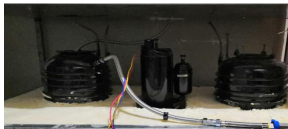
Figure: compressor fitting.
