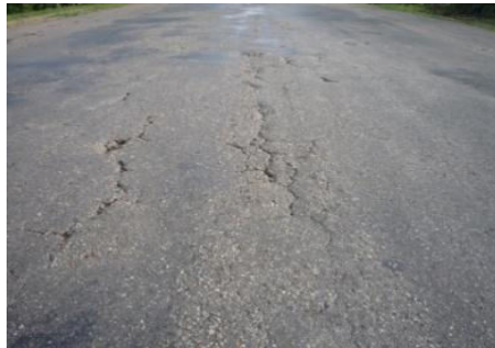
Fig 3.2 Existing Pavement of Longitudinal Cracking.
