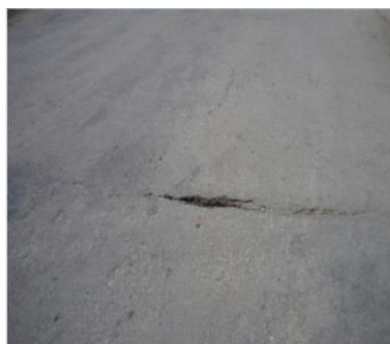
Fig 3.3 Existing Pavement of Transverse Cracking.
