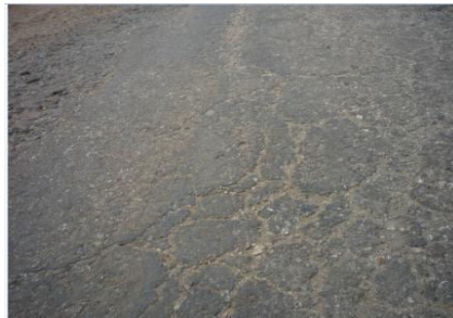
Fig 3.1 Existing Pavement of Alligator Cracking.
